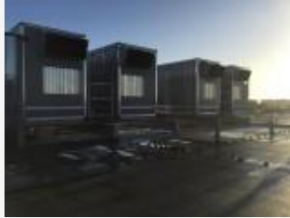
Primary air is being circulated through Switch Datacenters technology and air handling units (photo) on the rooftop
